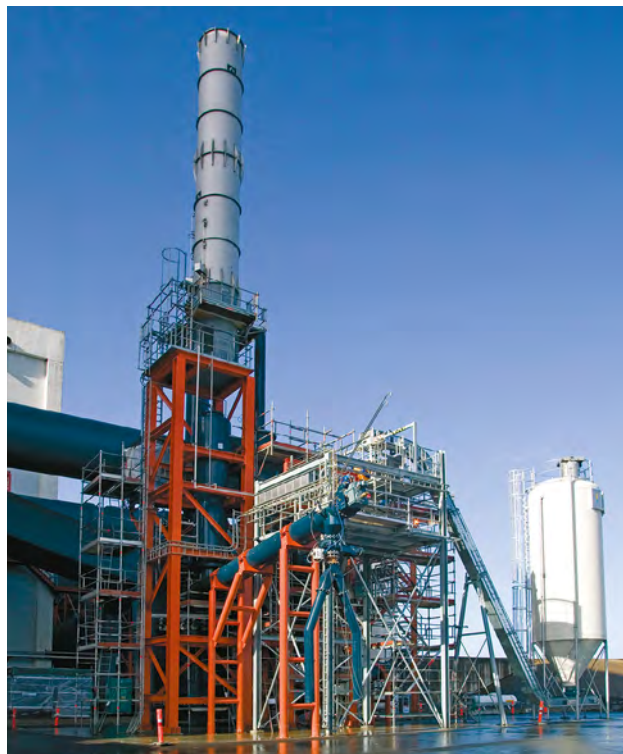
The Pyroneer gasification plant in Kalundborg. PHOTO Torben Skøtt, BioPress.
