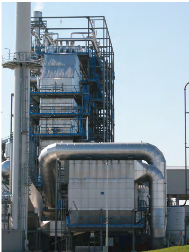
Versalis' €165 million industrial-scale second-generation ethanol plant in the Crescentino, province of Vercelli, Italy. PHOTO Food & Bio Cluster Denmark.
