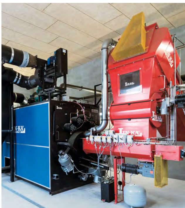
800 kW automatic plant from Linka Energy. PHOTO Linka Energy.
